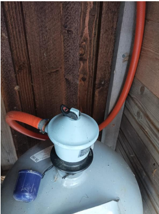
Main gas valve, open now turned to left and fire is visible.
